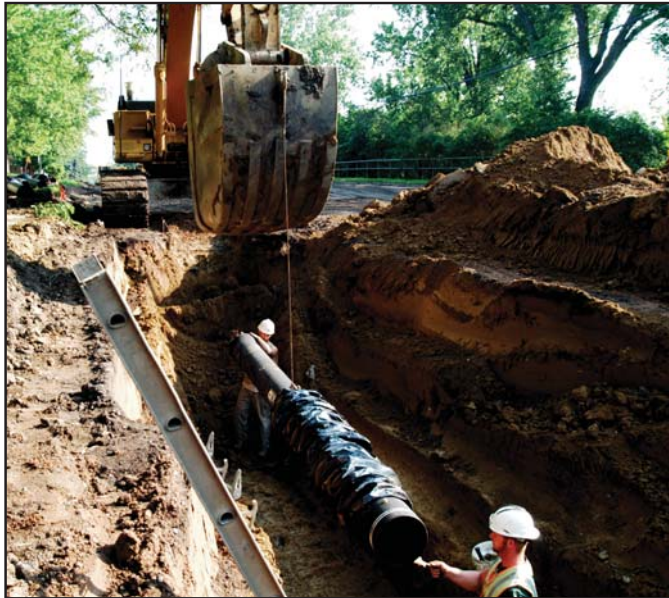
Construction workers lower a section of new ductile iron water main into place along the west side of Winnetka Avenue. The new water main is replacing deteriorated cast iron water main.
