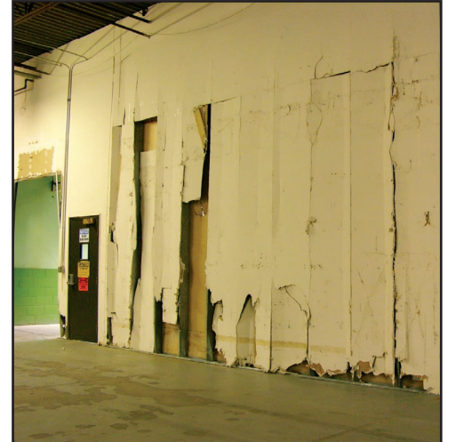
Before the renovation by Hillcrest Development, 5121 Winnetka was in disrepair and had significant lead contamination.
